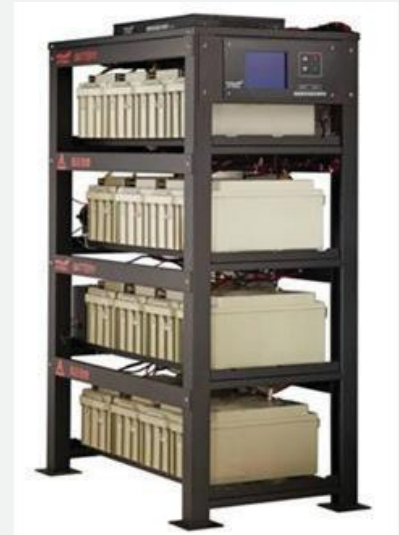
Battery cabinet and monitor system
